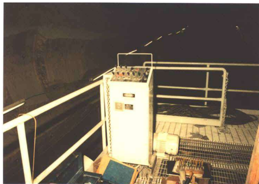
Here's a roof bolter and overhead crane control pedestal I installed on the mining machine in the Lanigan Potash mine!
